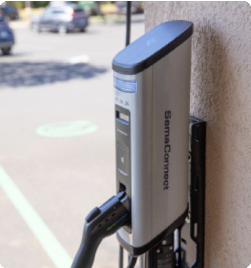
EV CHARGING STATION AT NAPILI PLAZA
