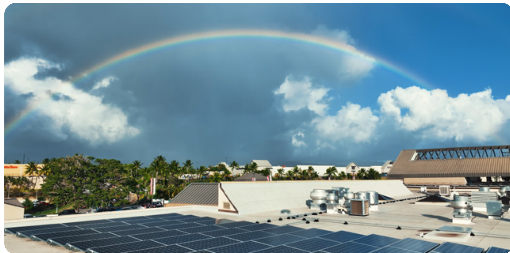
ROOFTOP SOLAR AT PEARL HIGHLANDS CENTER (PEARL CITY, O’AHU)
