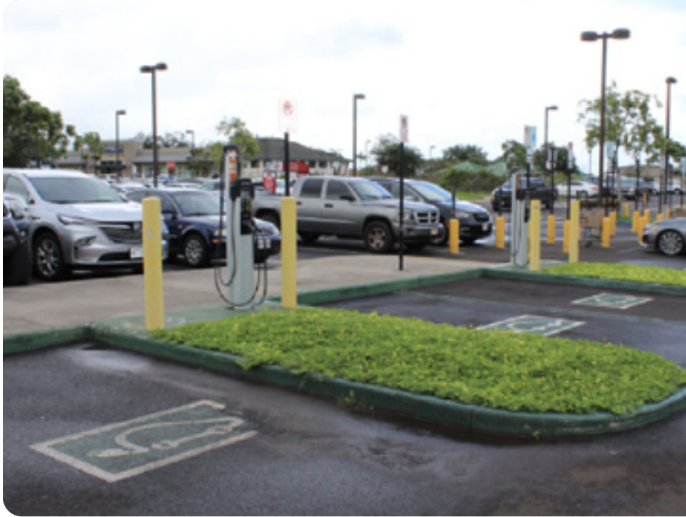
EV CHARGING STATIONS AT HOKULEI VILLAGE
